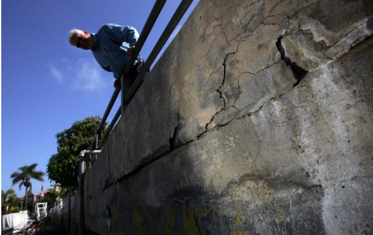
A sea wall in Naples Island, California shows signs of degradation. Salt air is one of a number of factors that can shorten the lifespan of concrete. Credit: Bob Chamberlin/Los Angeles Times/LA Times via Getty Images
