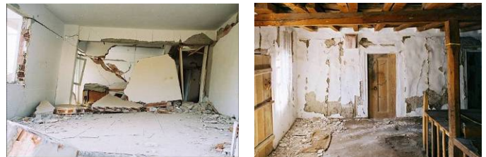
Fig 7 left: A view of a collapsed infill masonry wall in a reinforced concrete building in Gölçük, Turkey after the 1 st 1999 earthquake, showing how the brittle masonry wall can collapse out of the concrete frame soon after it begins to crack when the frame deforms from the earthquake forces. right: A view of a humus construction wall showing how the timber frame has held the masonry panels in place for the duration of the earthquake, despite the shedding of the plaster surface.
