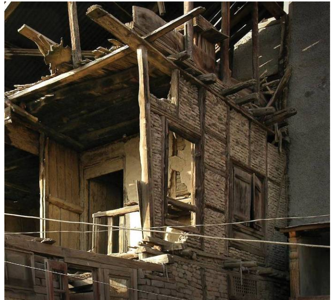
Fig. 2 Detail of dhajji dewari construction in a building under demolition in Srinagar, showing the timber frame, with the single-layer brick masonry infill. The walls are thin and light, when compared to bearing wall masonry. Notice how the floor joists are sandwiched between timbers at the floor level. This gives a strong friction connection between the floor diaphragms and the walls.
