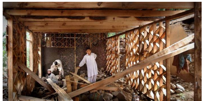
Fig. 5 New house being constructed in dhajji dewari by owner-builder in Pakistan Kashmir after the 2005 earthquake destroyed the prior house, which was of unreinforced rubble stone masonry. This family embarked on this construction after seeing that the one house to survive in the village was of dhajji construction. At the time they began construction, the Pakistan government would only provide reconstruction assistance for concrete construction, but one year after the earthquake, the government approved dhajji construction for assistance.
