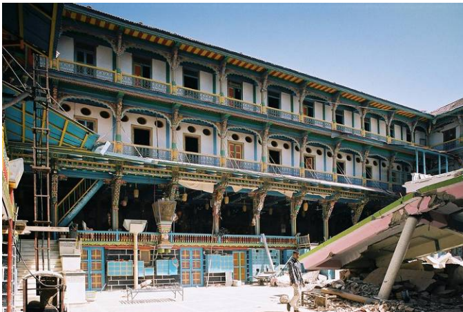
Fig. 4 This building in the Bhuj branch of the Ahmedabad-based Swaminarayan Temple is located in the heart of the walled city of Bhuj, yet it survived almost undamaged, while the modern concrete pavilion seen on the right collapsed. The construction is of timber frame with masonry infill, like that otherwise common in Ahmedabad, but rare in Bhuj.
