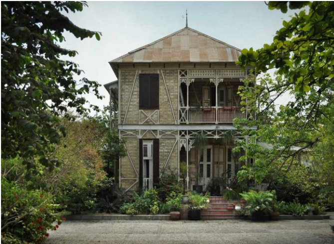
Fig. 10 A late 19 th century house of colombage construction in Port-au-Prince after the 2010 earthquake. This house, despite its age, suffered only minor damage. Colombage is the French word for timber frame with infill masonry construction, similar to that found in Turkey, as well as in India in Srinagar and Ahmedabad.
