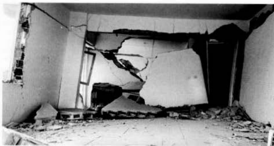
Fig. 13. The infill wall in this reinforced-concrete building in Turkey offered little resistance once it began to crack in the earthquake, unlike the timber-laced walls of the hımış construction.
