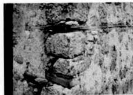
Fig. 3. Detail of lower-story walls showing hatıllar imbedded in wall, and lapping at the corners, in Safranbolu, Turkey.
