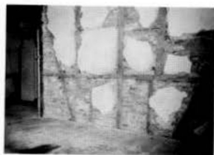
Fig. 8. Damaged interior wall exposing an undamaged brick infill wall behind, in Düzce, Turkey. The plaster cracking and falling at the edges of the panels, where the wood intersects with the brick, is characteristic of the damage to the hımış style of construction. This is a more extreme example of plaster shedding.
