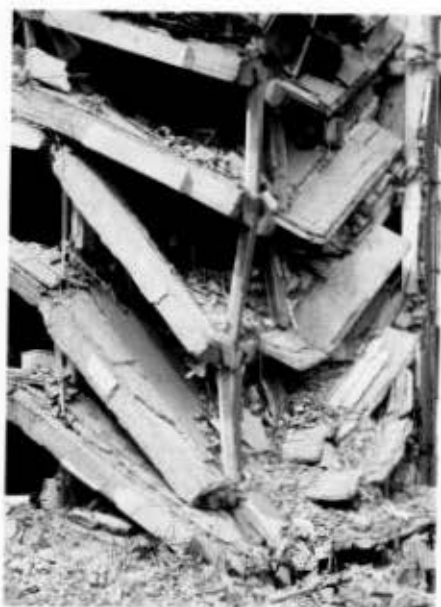
Fig. 6. Gölcük. Partially collapsed reinforced-concrete apartment house.
