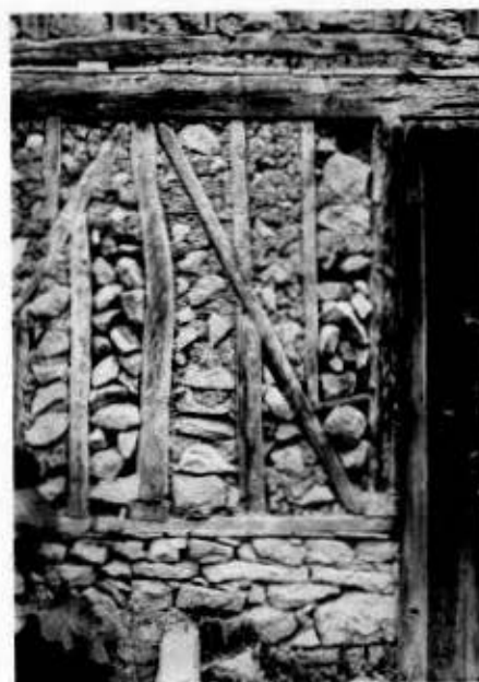
Fig. 2. Hıms -style wall with stone infill laid in mud mortar, in Safranbolu, Turkey.
