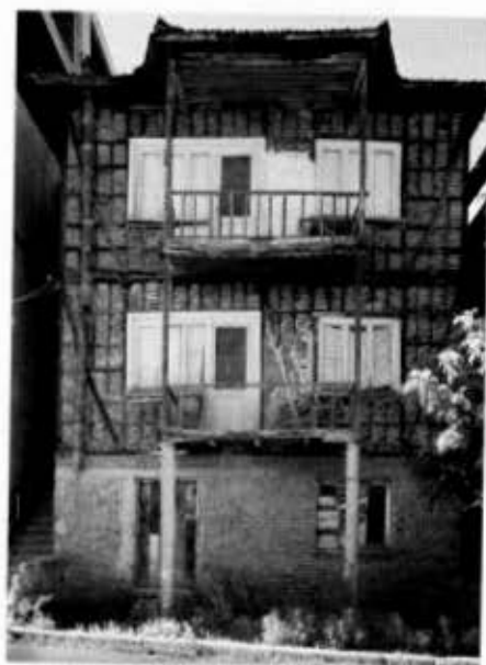
Fig. 7. Hımış house that survived the earthquake with no visible damage to its exterior in the heart of the damage district in Gölcük, Turkey.
