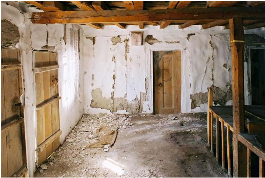
Figure 13: Interior of himiş house in Orta after earthquake showing damage to mud and lime plaster over infill walls.
