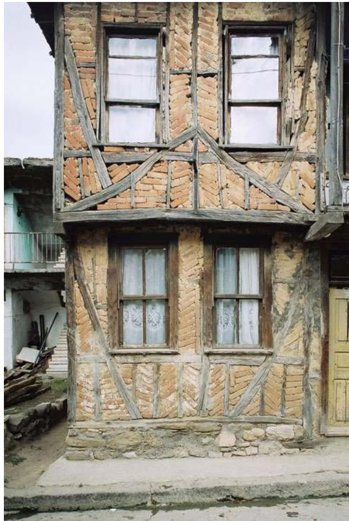
Figure 11: Hımış house in Gölcük after earthquake constructed in 1955. There was only slight damage to the interior of this house.
