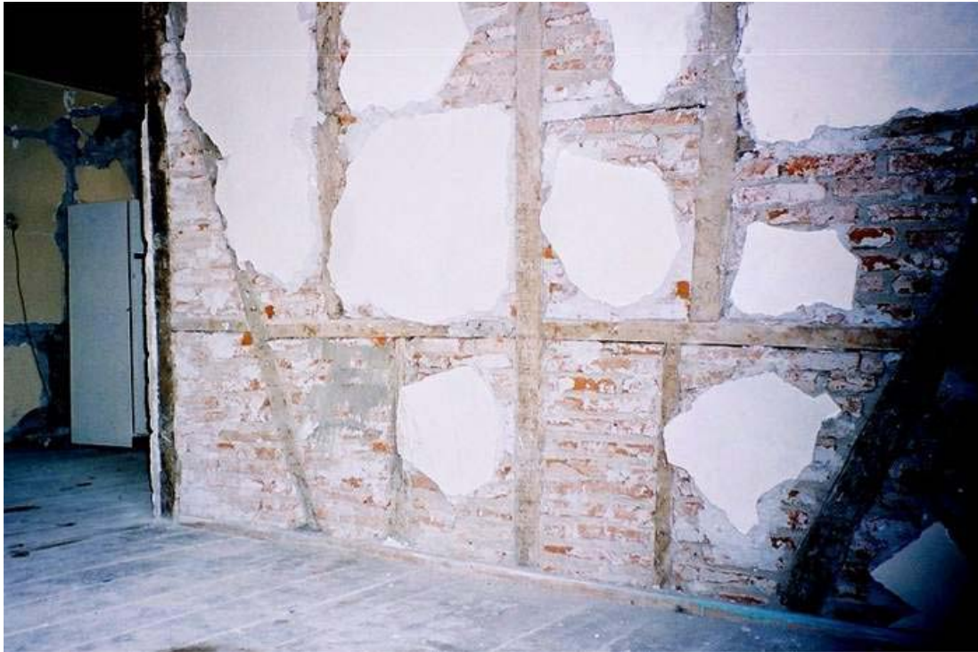
Figure 12: Himiş interior wall in Düzce after earthquake.
