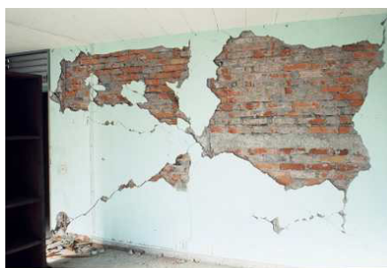
Figure 31: Infill RC building in Mexico City after the 1986 earthquake collapsed many buildings nearby. Each panel is subdivided vertically and horizontally.
