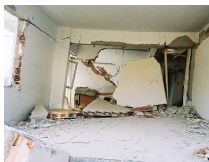
Figure 14: Soft-story collapse of a RC infill wall building in Adapazzari where the infill walls resisted the pancake collapse of the upper floors.
