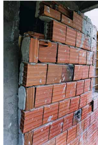
Figure 29: Infill wall RC building in Mexico City damaged in 1985 earthquake. The infill masonry in this structure almost caused the collapse of the building. The damage to the corner column that left the building teetering on the edge of collapse can be seen on the right.
