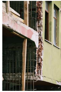
Figure 27 & 28: Five story building damaged in the 1999 Düzce earthquake in Turkey, being retrofitted with reinforced concrete shearwalls. No.28 shows the existing hollow clay block walls removed and steel being inserted for the construction of a reinforced concrete shearwall. These images illustrate the extent of the work, and disruption needed for earthquake strengthening using shearwalls. The occupants had to move out for the duration of this work as many existing walls were removed.
