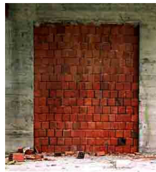
Figure 23: Typical Turkish RC building under construction showing the hollow block infill being installed.
