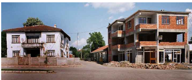
Figure 9: Three story RC building next to a 2½ story himiş house near Düzce showing the repair of severe damage to the RC building (notice the size of the ground floor columns). The himiş structure has lost only stucco on the side. Almost all of the hollow clay block on the RC building has been reconstructed after the earthquake. This shows that even low rise RC buildings sometimes suffered more damage than nearby traditional buildings.
