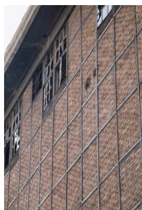
Figure 33: Detail of masonry wall in Istanbul’s Silahtarağa Powerplant showing brick infill with horizontal and vertical light-frame steel “I” sections. (Kıraç et al, 2003) This construction is similar to that shown in Figure 34 below.
