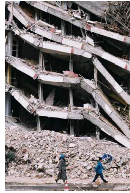
Figure 1: “Pancake” collapse in Mexico City, 1985.
