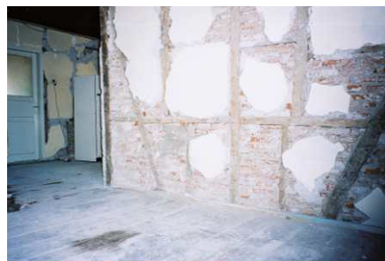
Figure 12: House in Orta, Turkey one day after the 2000 Orta earthquake – showing plaster cracking that reveals the timber frame.
