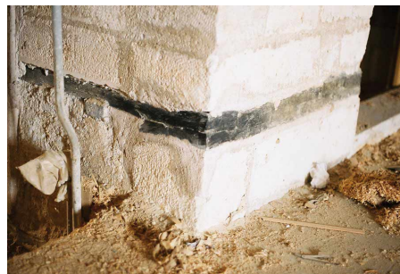
Figure 5: LEFT: Interior of Ancient Caravansary in Safranbolu with hatıl visible along right wall.
