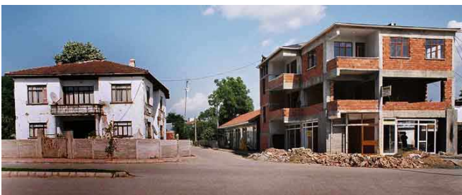
Figure 17: Three story RC building next to a 2½ story himiş house near Düzce showing the repair of severe damage to the RC building (notice the size of the ground floor columns). The himiş structure has lost only stucco on the side. Almost all of the hollow clay block on the RC building has been reconstructed after the earthquake. This shows that even low rise RC buildings sometimes suffered more damage than nearby traditional buildings.
