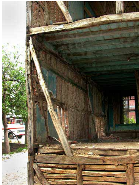
Figure 11 & 12: Partially demolished house in Golcuk showing the single brick wythe thickness of typical himış wall. On the LEFT is the exterior and on the RIGHT is the interior face of the same wall.
