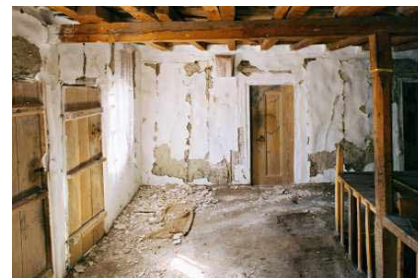
Figure 22: LEFT: House in Orta, Turkey one day after the 2000 Orta earthquake – showing plaster cracking that reveals the timber frame.
