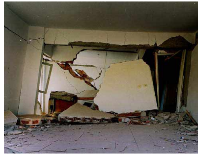
Figure 20: Hımış interior wall in house in Düzce earthquake damage district showing “working” of wall that caused loss of plaster.
