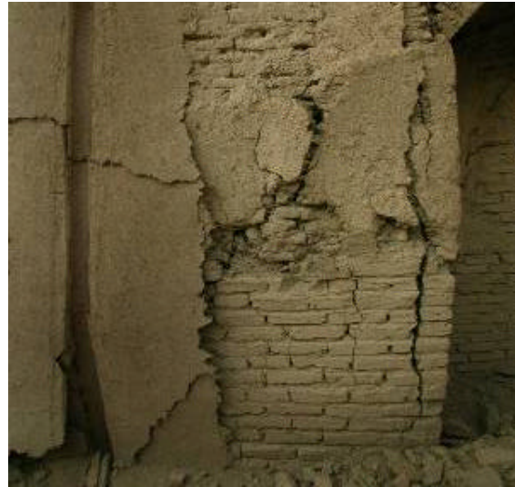
Figure 8: Pier in a partially collapsed section of the Caravansary showing the bursting of the outer layers from internal expansion from the earthquake vibrations.
