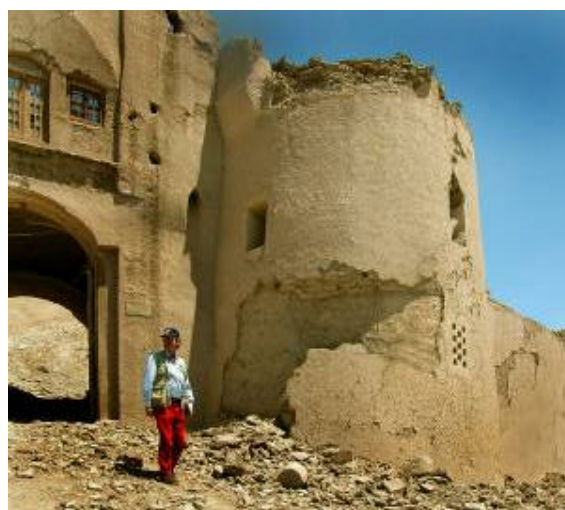
Figure 15: One of the few surviving turrets has a room in its base, as shown by the ground floor window. The floor diaphragm timbers extend through the walls, and are now visible after the stucco fell off. The collapsed masonry and stucco is from what appears to be a modern-day modification of the shape of the tower in the tradition of Viollet-le-Duc. The tower's original surface underneath is intact.
