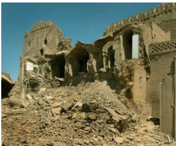
Figure 14: Buildings above the Stables courtyard that collapsed from the lateral spreading failure of the retaining wall and fill beneath.
