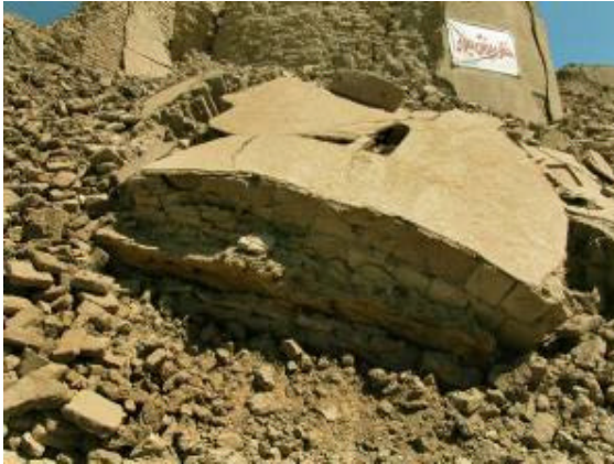
Figure 22: Collapsed section of the main gateway showing imbedded timber reinforcement of the Khesht wall.
