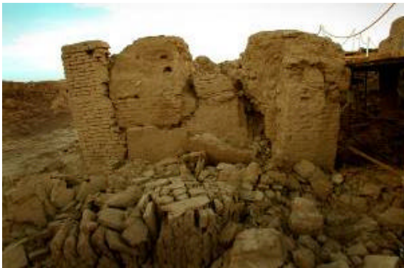
Figure 17: A massive pier composed of different periods and types of Khesht and chineh construction that have separated from each other during the earthquake.
