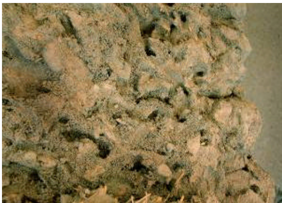
Figure 2: Evidence of termite damage in a wall of the Arg-e Bam showing extensive deposits of frass with insect tunnels.
