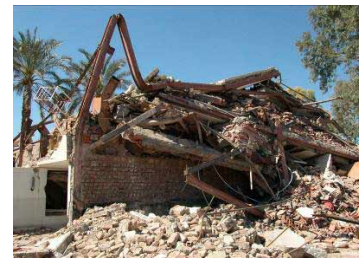
Fig.3 Collapsed steel frame infill wall building in 2004 Bam, Iran earthquake.
