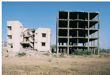
Fig.2 Bare Frame of incomplete building next to partial collapse in 2001 Gujarat earthquake.
