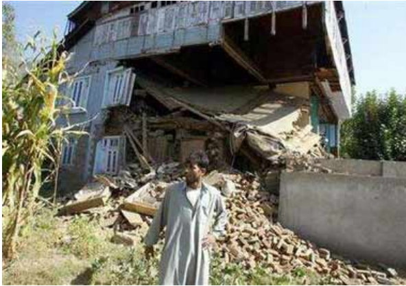
Fig.10 House in Baramulla, Kashmir, Oct.8,2005. The roof and 3 rd floor walls were left in place with no support from below. The intact walls of the top floor are of timber with masonry infill (Dhajji Dewari) construction, while the destroyed lower floors are unreinforced masonry without the timber armature. (Reuters) See (Langenbach, 1989) for more on Dhajji Dewari.
