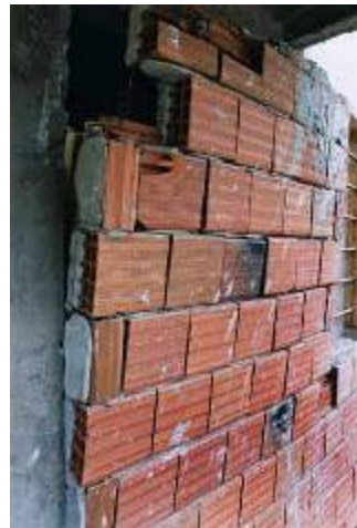
Figure 26: Infill wall RC building in Mexico City damaged in 1985 earthquake. The infill masonry in this structure almost caused the collapse of the building. The damage to the corner column that left the building teetering on the edge of collapse can be seen on the right.
