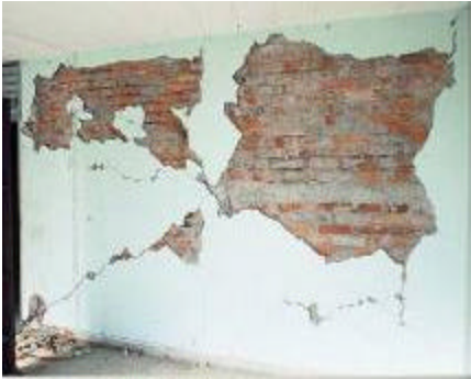
Figure 32: Infill RC building in Mexico City after the 1986 earthquake collapsed many buildings nearby, including the one in Figure 20. Each infill wall is subdivided vertically and horizontally into 4 panels.
