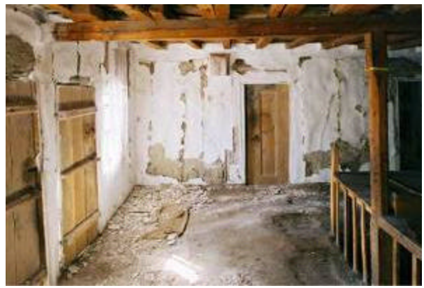
Figure 46: RIGHT: Interior of himis house after the Orta earthquake showing the “working” of the masonry panels. This view shows the inherent flexibility of the structures, but the inevitable disruption of the mud and lime plaster leads people, including both the owners and the government inspectors to assume that the buildings has lost strength when it has not.
