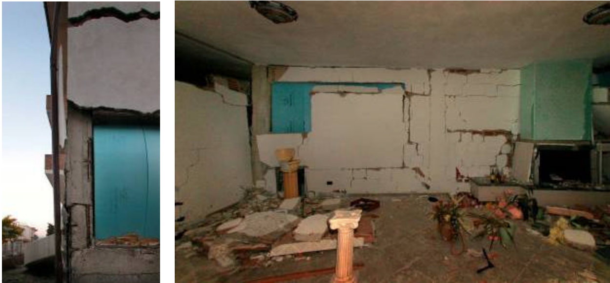
Figure 49 & 50: Interior and exterior of a damage reinforced concrete building in San Giuliano di Puglia after the Molise earthquake illustrating that the frame is on the verge of collapse. While this building will be difficult or impossible to repair to an earthquake-safe condition, the traditional house in Orta in Figure 46, with a similar amount of debris on the floor has lost a negligible amount of its total capacity, and can be easily repaired.
