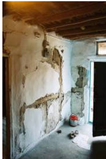
Figure 47: Interior vestibule of house in Adapazari after the 1999 Izmit earthquake.
