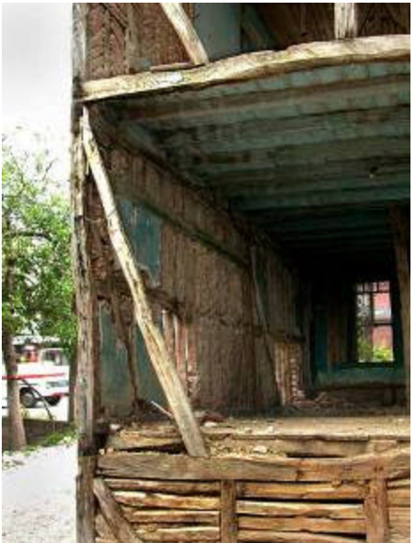
Figure 41: Partially demolished house in Golcuk showing the single brick wythe thickness of typical himis wall. On the LEFT is the exterior and on the RIGHT is the interior face of the same wall.
