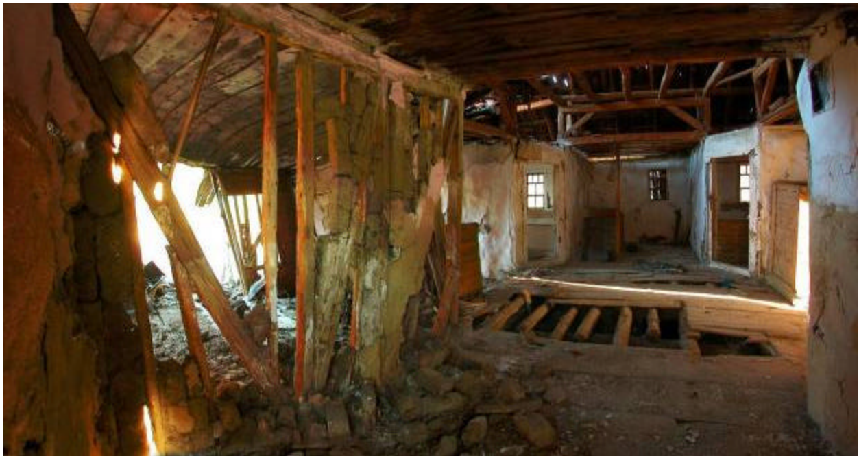
Figure 65: This house in Eden had been abandoned for years before the earthquake. Despite its deteriorated condition, the earthquake damage was limited to the collapse of some of its walls. The basic rough construction characteristic of a rural area without a saw mill or access to a kiln can be seen with the undressed logs used for the structure, and unfired adobe blocks used for the infill.
