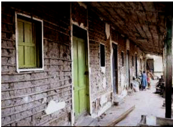
Figure 17: Bahareque construction in San Salvador showing effects of 1986 earthquake. The loss of the stucco shows that the wall underwent deformations without loss of its underlying structural integrity.
