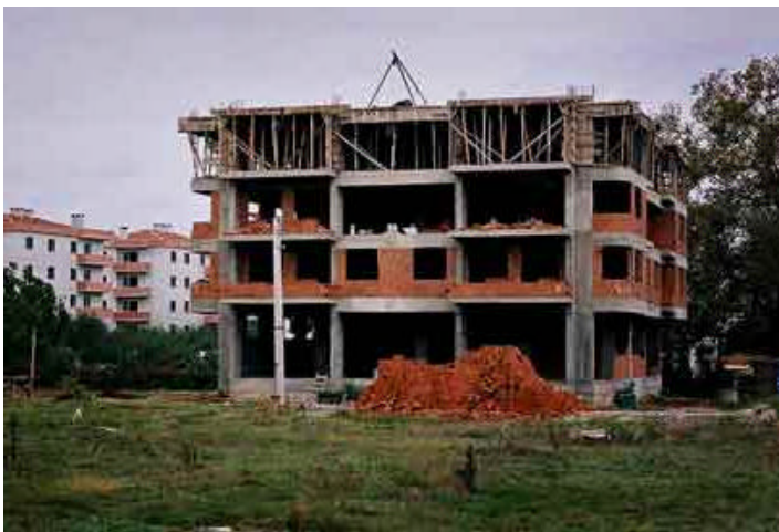
Figure 22: Typical Turkish RC building under construction showing the hollow block infill being installed.
