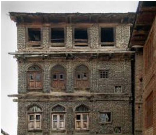
Figure 15: Example of Taq construction in Srinagar, Kashmir, 2005. The timbers in the masonry walls only run horizontally parallel to the wall and through the wall.
