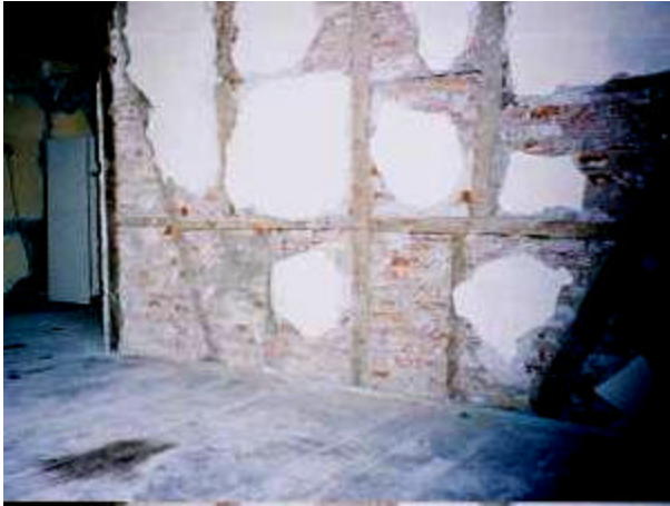
Figure 36: Himis interior wall in house in Düzce earthquake damage district showing “working” of wall that caused loss of plaster.
