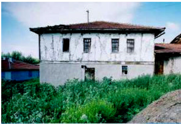
Figure 45: LEFT: House in Orta, Turkey one day after the 2000 Orta earthquake – showing plaster cracking that reveals the timber frame. There was no evidence of damage beyond that of the cracked plaster.
