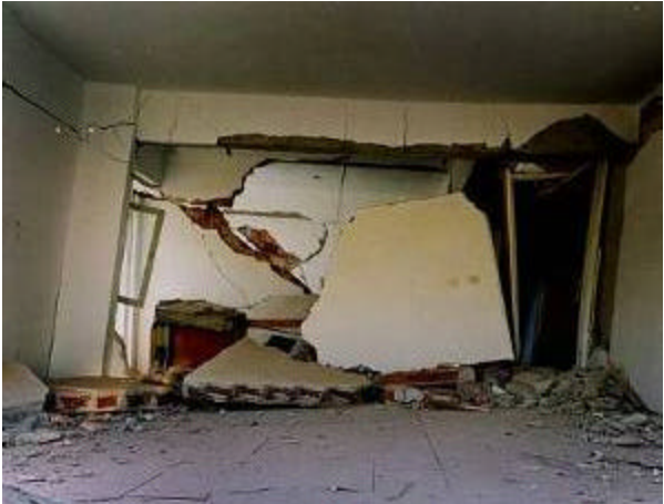
Figure 37: Collapse of a brittle interior hollow clay block wall illustrating typical failure pattern for such walls lacking subdivisions.
