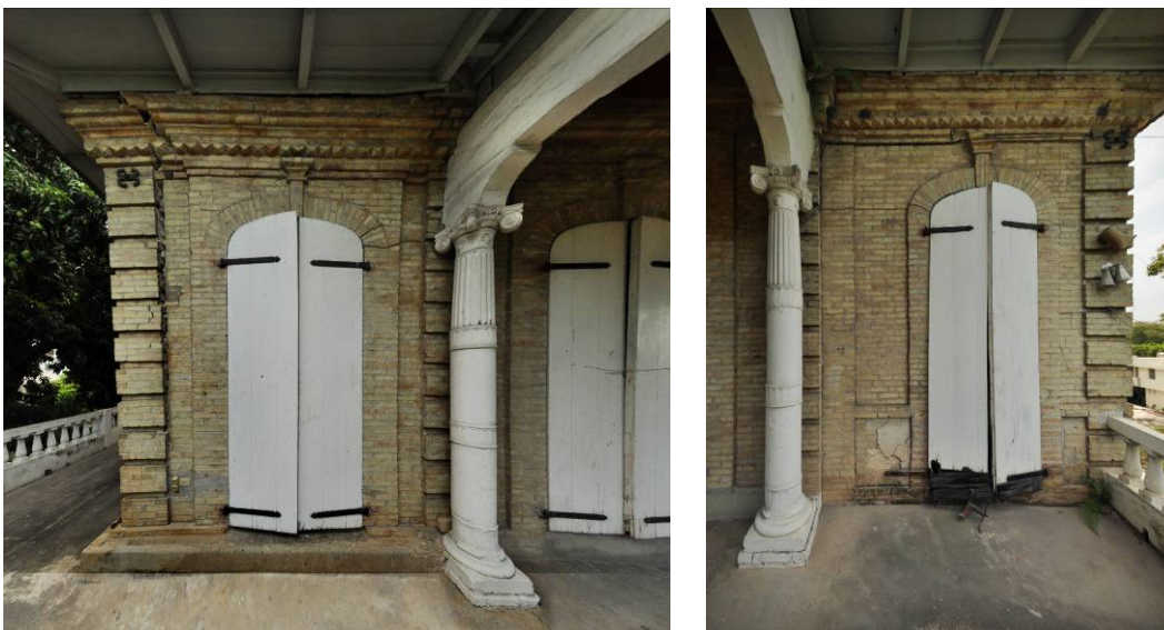
Figure 8. 2nd storey wall of a masonry house showing the iron brackets that connect the through wall steel ties that form a continuous ring around the house. The left view shows the wall deflected outward because the plate was missing on the wall around the corner, whereas the view of right hand end of the same wall shows no visible damage because the plate was still attached and thus effective in preventing the spreading.
