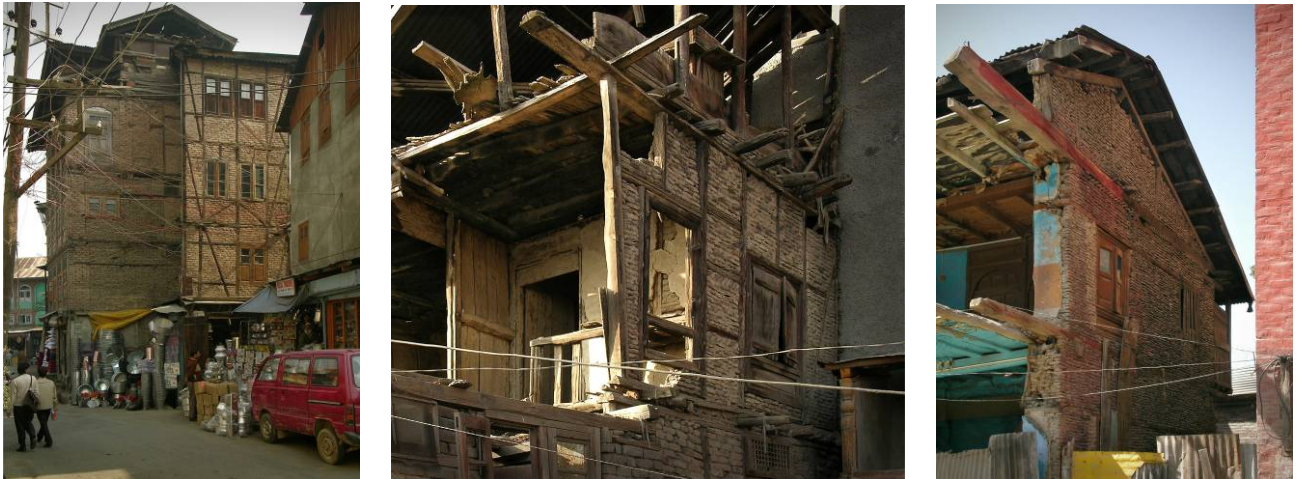
Figure 2. Buildings in Srinagar, Kashmir. left: The building on the left is of taq timber laced bearing wall construction, and on the right is of dhajji dewari construction. middle: A partially demolished dhajji dewari building showing timber frame with infill masonry construction. right: A partially demolished building showing timber-laced masonry bearing wall typical of taq construction.
