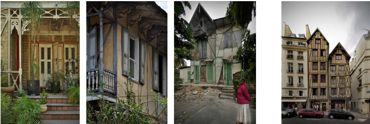
Figure 5. The three photos on the left show pan-de-bois houses in Haiti. The left view shows brick infilling, the middle, with stucco over rubble stone, and the right shows a house that was heavily eaten by termites, yet which survived. The interior timber cladding is visible where the infill stone has fallen. The right hand view shows medieval pan-de-bois houses in Paris with their steeply gabled roofs.
