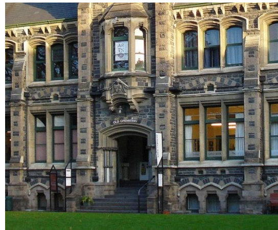
Figure 22. Detail showing the exterior steel rods and clamps that are part of the retrofit done during the 1980's. This retrofit was comparatively less expensive than other methods where new structural frames were added.
