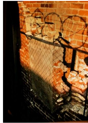
Figure 28. The concrete infilling of this former window opening was forced out of the wall during the 1994 Northridge earthquake in Los Angeles, Ca. USA.
