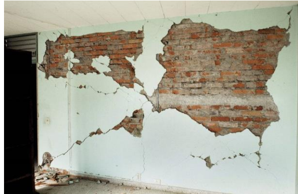
Figure 14. View of an infill wall in the building in Fig. 13. The fallen plaster has revealed that the wall was reinforced with an RC sub-frame that kept the masonry from falling out of the frame, and thus helped prevent a pancake collapse of the upper floors, saving the lives of the occupants. (See Section 2.10 below)
