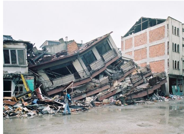
Figure 6. A typical view of a pancake collapse of a 5 story reinforced concrete infill masonry building in Adapazari, Turkey after the 1999 Kocaeli Earthquake.
