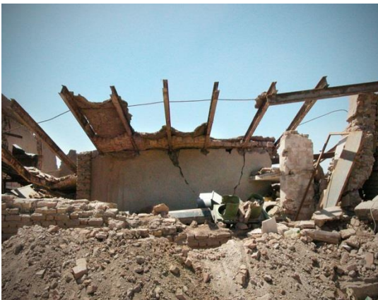
Figure 10. Collapsed building with adobe walls and steel and fired brick jack arch roof in Bam, Iran after the 2003 earthquake.
