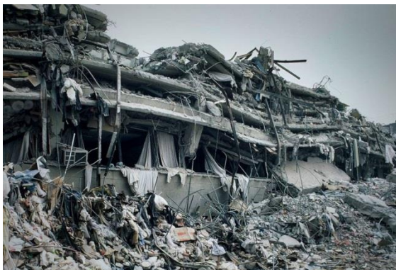
Figure 31. View of the Juarez Hospital after the 1985 Mexico City earthquake collapsed it trapping approximately 950 people, of which 561 were killed.
