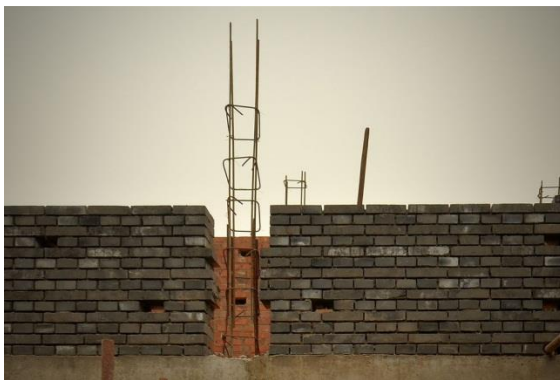
Figure 17. Typical detail of 'confined masonry' when under construction before the walls are topped out and the columns are poured. This example was photographed in Beijing, China.
