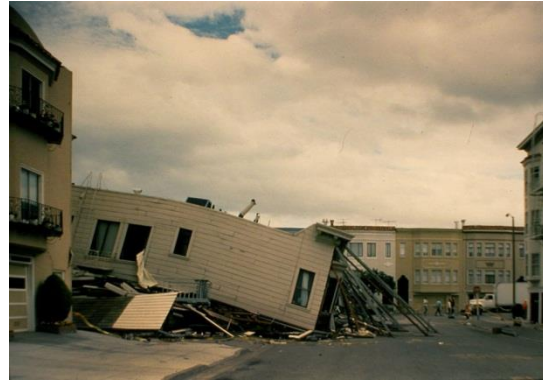
Figure 10. Collapsed timber framed multi-story apartment house in San Francisco after the 1989 Loma Prieta earthquake. There were only 3 fatalities in this earthquake caused by the collapse of timber frame buildings.
