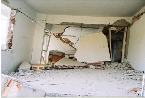
Figure 29. View of a collapsed infill masonry wall in a partially collapsed multistory building in Gölcük, Turkey after the 1999 Kocaeli earthquake. This kind of damage is typical when the infill walls are single layers of brittle masonry set in cement mortar without any sub-frame or other reinforcement.
