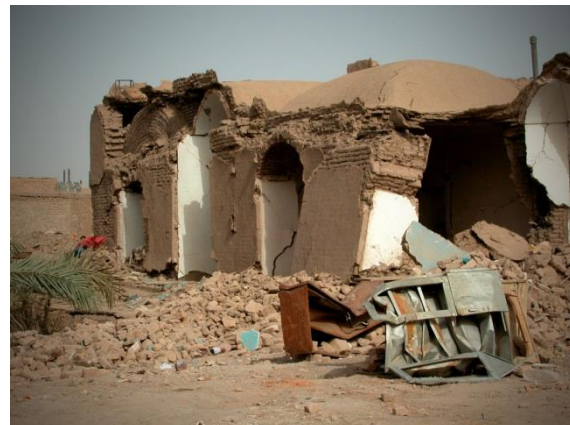
Figure 11. Partially collapsed adobe building of traditional unreinforced construction in Bam, Iran with most of its vaulted roofs still standing.
