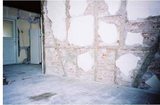
Figure 30. View of the typical timber frame with masonry infill of Turkish hıms construction. This photo was taken in a two and a half story dwelling in Düzce, after the 1999 Düzce earthquake. It was surrounded by collapsed RC multistory buildings. It is this kind of construction that forms the inspiration for the “Armature Crosswalls” concept.
