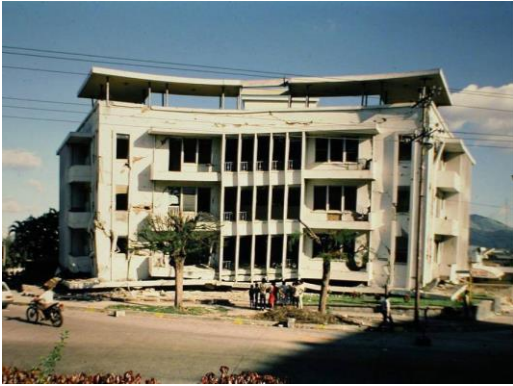
Figure 13. This was a 5 story RC frame building after the 1986 San Salvador earthquake caused a soft-story collapse. Figure 14 was taken in one of these remaining floors.
