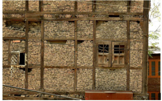
Figure 8. Example of dhajji dewari construction in Srinagar. This is an example with only rectangular panels. There is often in the present a belief that diagonals are necessary, just as they were in Lisbon in the gaiola that was invented after the 1755 earthquake, but there is increasing evidence that they are not necessary, and may even be counter-productive (Credits: Randolph Langenbach).
