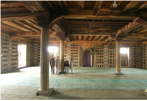
Figure 7. Example of cribbage construction, The Khankah in Pampore, near Srinagar, ca. 1600. When photographed in 2007, the interior was being clad with plywood in order to, as they stated, to “modernize” the interior (Credits: Randolph Langenbach).
