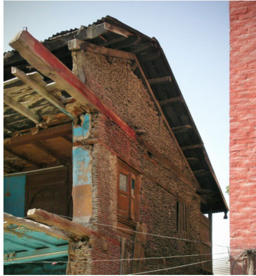
Figure 6. A three and a half story building in central Srinagar, Kashmir, India, of taq timber-laced construction partially demolished for a street widening (Credits: Randolph Langenbach).
