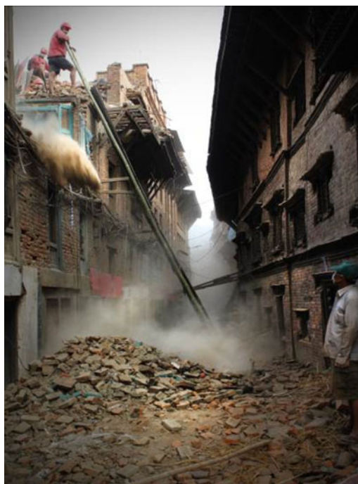
Figure 1. View of Bhaktapur, Kathmandu area, Nepal after the Gorkha Earthquake (Credits: Xavier Romão & Esmeralda Paupério).
