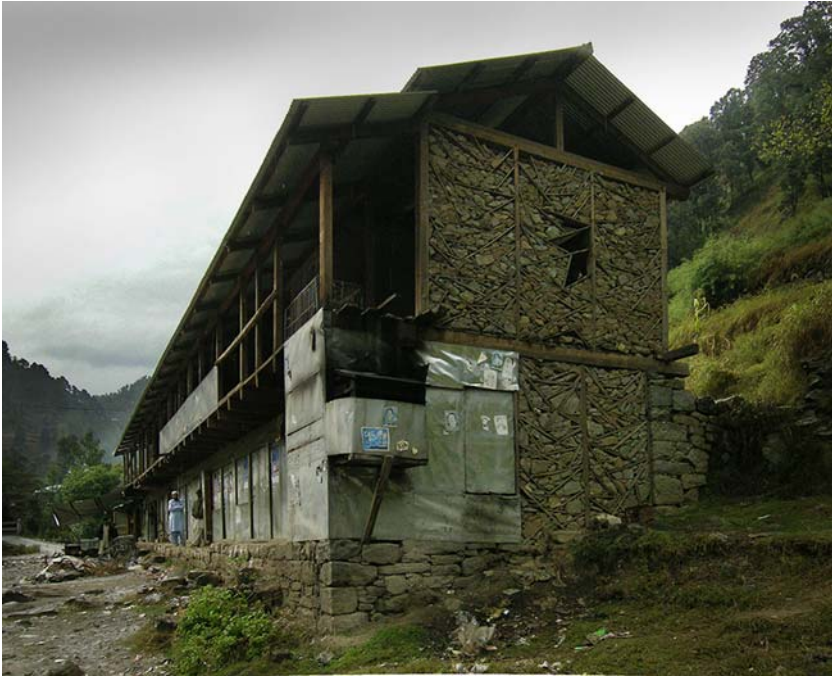
Figure 1.30 Dhajji-dewari building in rural Pakistan, Kashmir, after the 2005 earthquake, showing the few missing wall panels of infill masonry.
