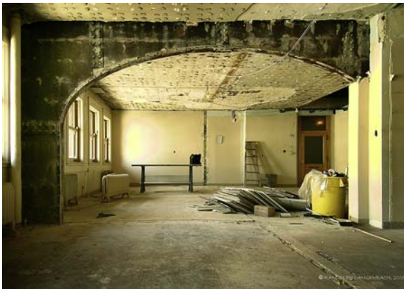
Figure 1.22 An office interior remodeling project in the south wing of the 1891–1893 steel-frame Monadnock Building in Chicago briefly revealed this view, an example of what Freitag defines as the “table leg” portal arch. The photograph was taken in 2005.
