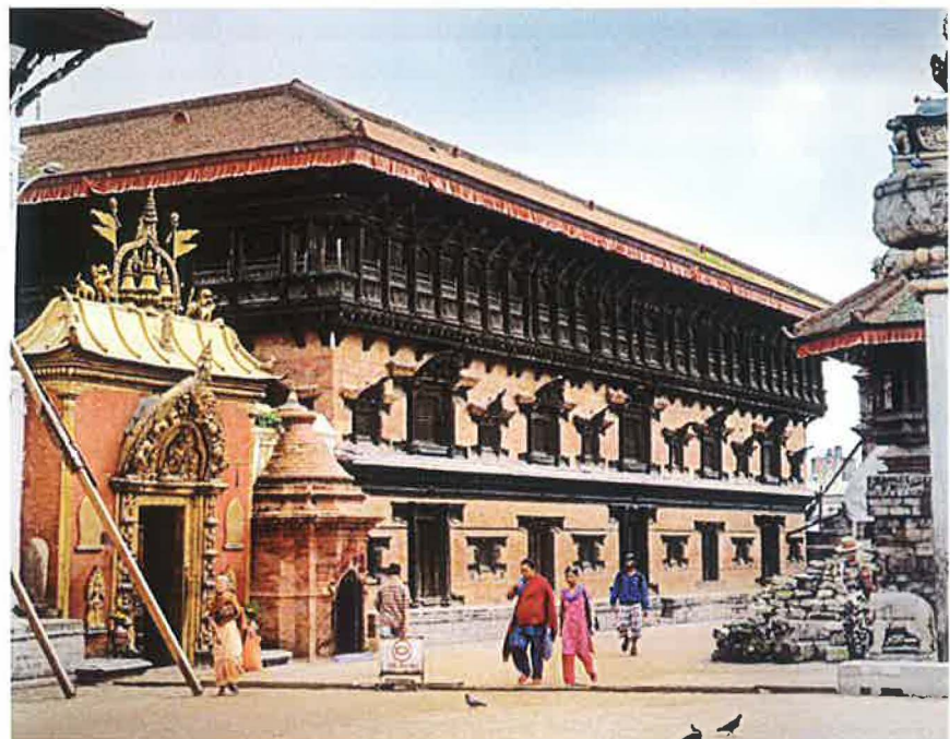
10 / Temple in Kathmandu, Durbar Square showing the brick wall with a convex bowing after the earthquake from the wedge shake bricks.
