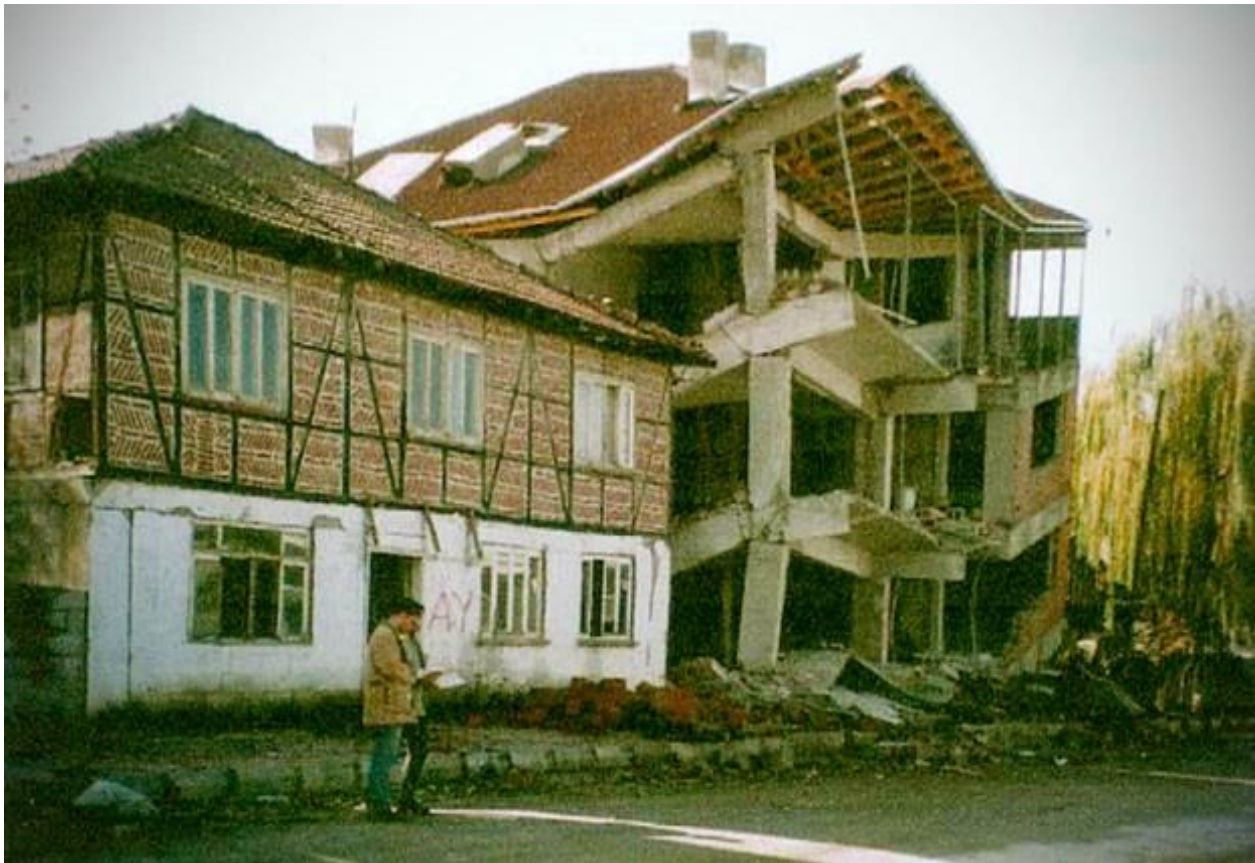
Figure 26: Formerly 4 story RC building next to dhajji building with very little damage from 1999 earthquake. (reproduced with permission from Adem Doğangün (Doğangün et al., 2006))
