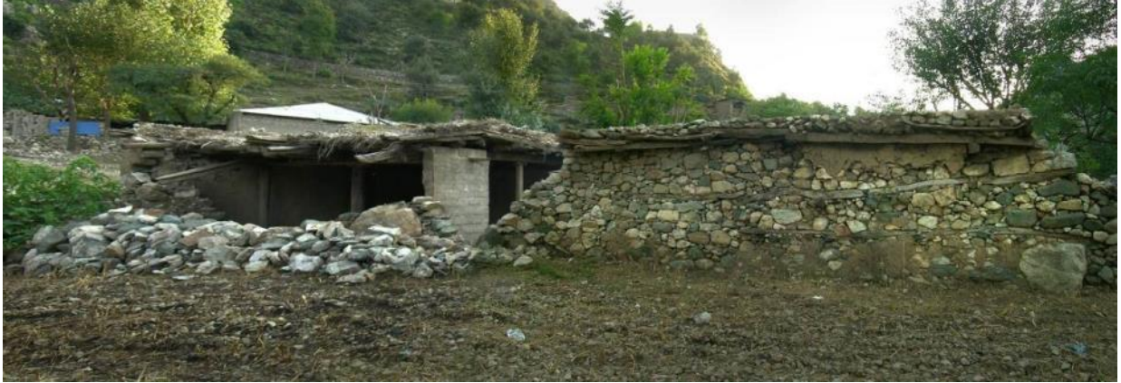
Figure 9: URM wall on left and bhatar wall on right after earthquake
