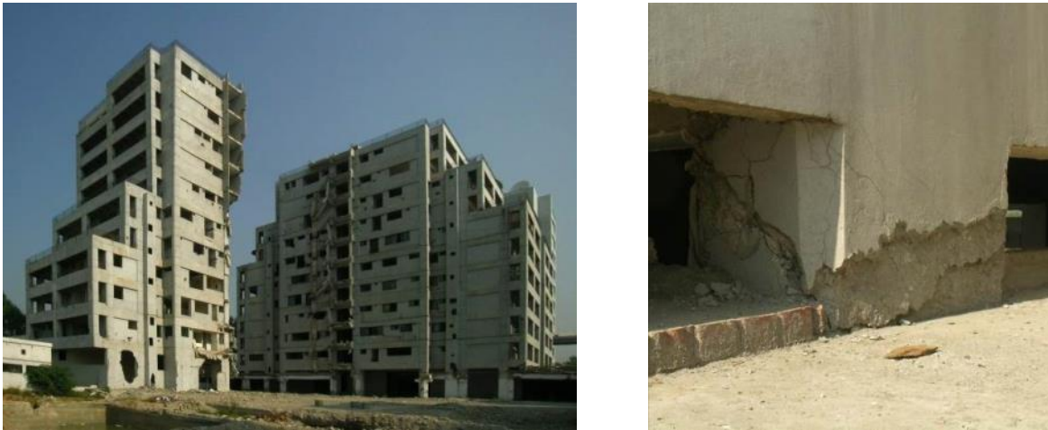
Figure 38: Margalla Towers, Islamabad (middle) after debris removal exposes the basement level 'soft story' and (right) base of the section next to that which collapsed showing evidence of onset of short column failure
