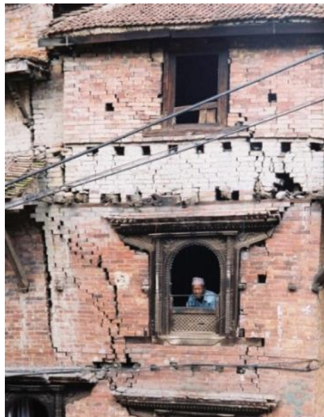
Figure 20: A similar sized building in Kathmandu, Nepal, showing effects of differential settlement without timber lacing causing the building to begin to split apart
