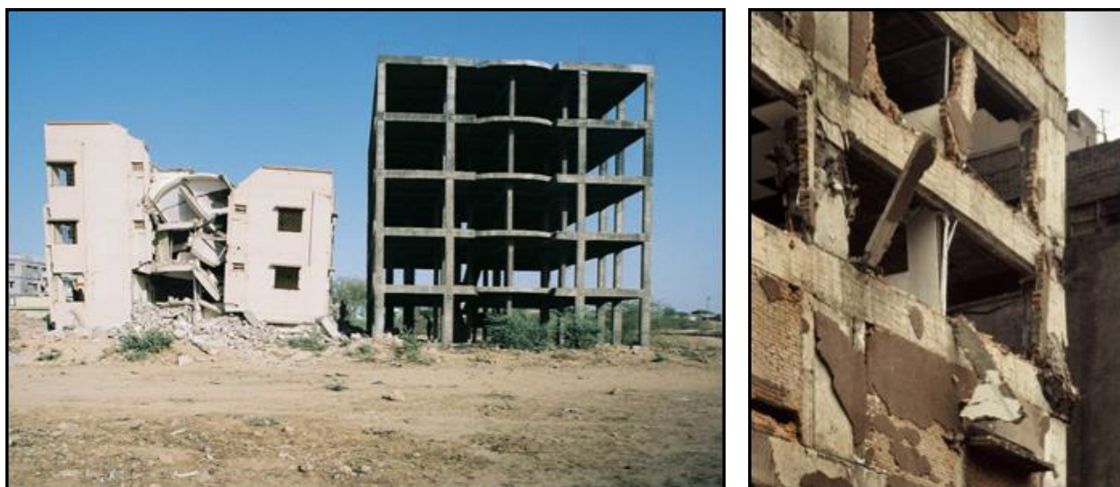
Figure 43: Buildings that were intended to be identical when finished, located near Bhuj, India after the 2001 Gujarat earthquake
