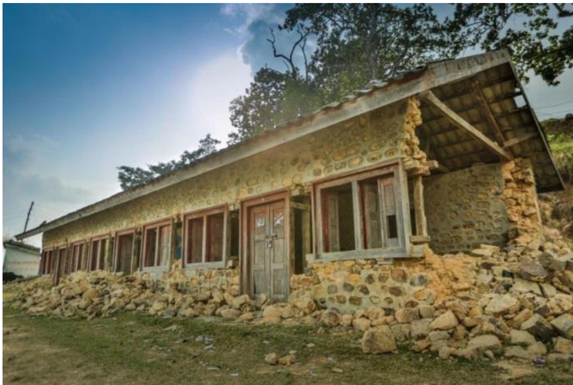
Figure 57: School building with front and rear walls still standing with a ceramic tile roof. (photos courtesy Nepal School Projects NGO)
