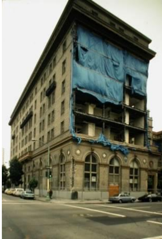
Figure 37: Hotel Oakland, Oakland, California after 1989 earthquake which caused much of this end façade to fall off
