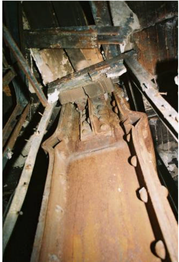
Figure 3: Buckled riveted steel column, 90 West Street
