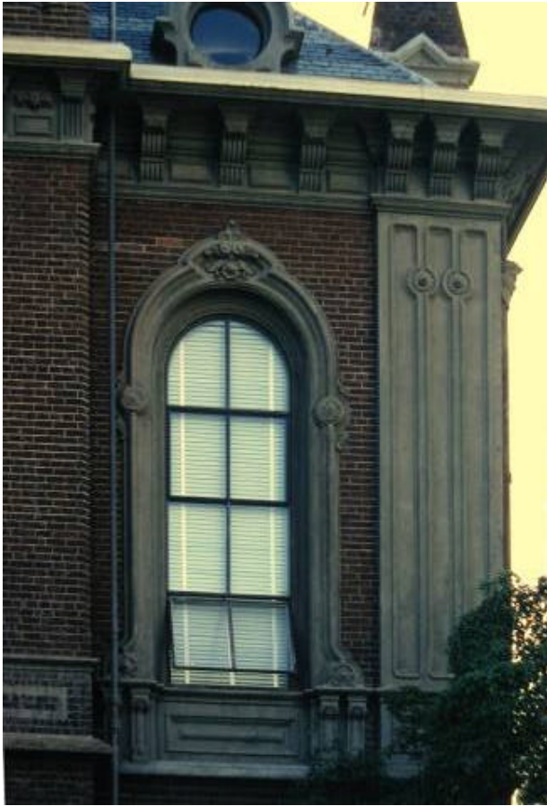
Figure 6C: Exterior of South Hall showing large ornamental cast iron corner bracket. The bond iron in the brick walls terminates at the large bosses.
