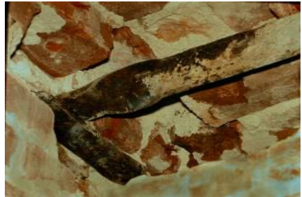
Figure 6A: Bond iron inside the brick exterior wall of South Hall exposed during construction work.
