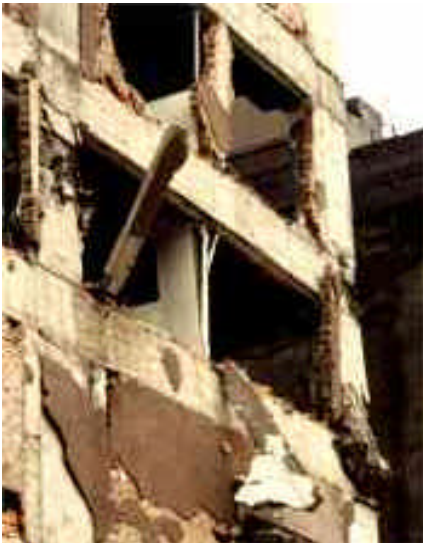
Victims of the 1985 Mexico City earthquake, the reinforced concrete columns on the right of this building have been damaged almost to the point of collapse by the "equivalent diagonal strut" effect of the infill masonry.
