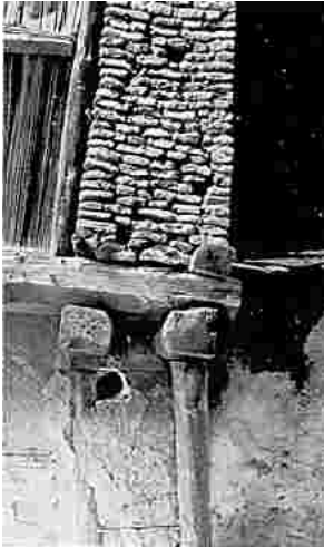
A typical masonry-wood connection in Kashmiri construction. These wood brackets are ubiquitous in both TAO and DHAJJI-DEWARI structures. The masonry simply rests on top of the wood beams.
