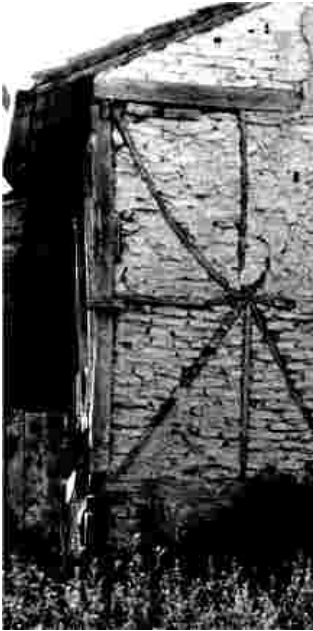
The brick-nogged construction shown here survived the great earthquake of 1963 in Skopje, Yugoslavia.
