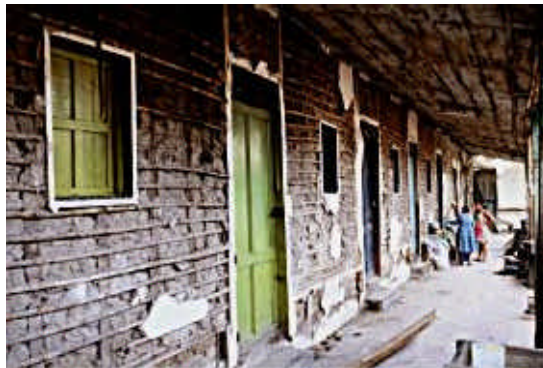
An example of BAHAREQUE construction, a native method in El Salvador, this building withstood the quake with little damage apart from plaster falling off the walls.
