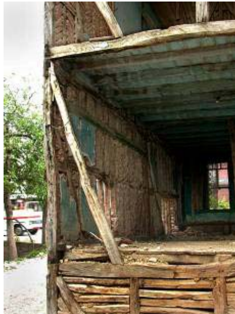
Figure 35: Partially demolished house in Golcuk showing the single brick wythe thickness of typical hımış wall. On the LEFT is the exterior and on the RIGHT is the interior face of the same wall.
