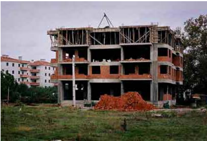
Figure 20: Typical Turkish RC building under construction showing the hollow block infill being installed.
