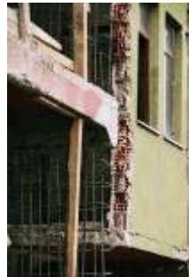
Figure 27 & 28: Five story building damaged in the 1999 Düzce earthquake in Turkey, being retrofitted with reinforced concrete shearwalls. No.30 shows the existing hollow clay block walls removed and steel being inserted for the construction of a reinforced concrete shearwall. These images illustrate the extent of the work, and disruption needed for earthquake strengthening using shearwalls. The occupants had to move out for the duration of this work as many existing walls were removed.
