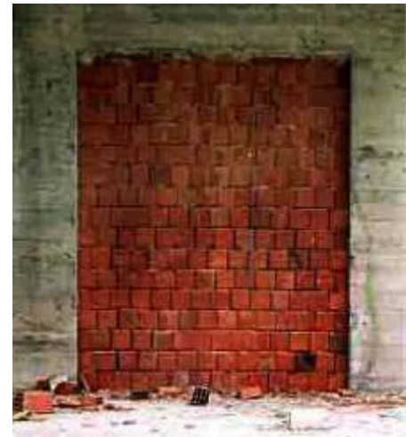
Figure 21: Typical hollow clay block infill as used in reinforced concrete residential construction in Turkey.
