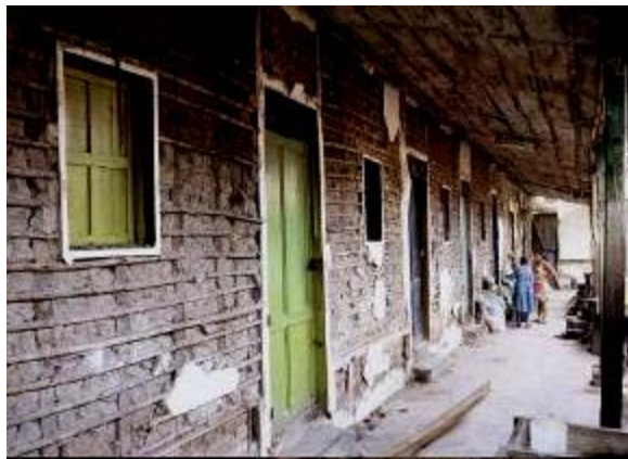
Figure 15: Bahareque construction in San Salvador showing effects of 1986 earthquake. The loss of the stucco shows that the wall underwent deformations without loss of its underlying structural integrity.
