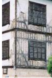
Figure 37: Large 3 story house in himış construction, Safranbolu, Turkey, 2000. Safranbolu is now on the World Heritage List because of its unique collection of intact Turkish vernacular houses.
